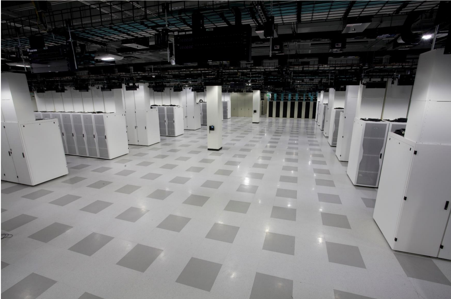
Cisco's Data Center in Texas
