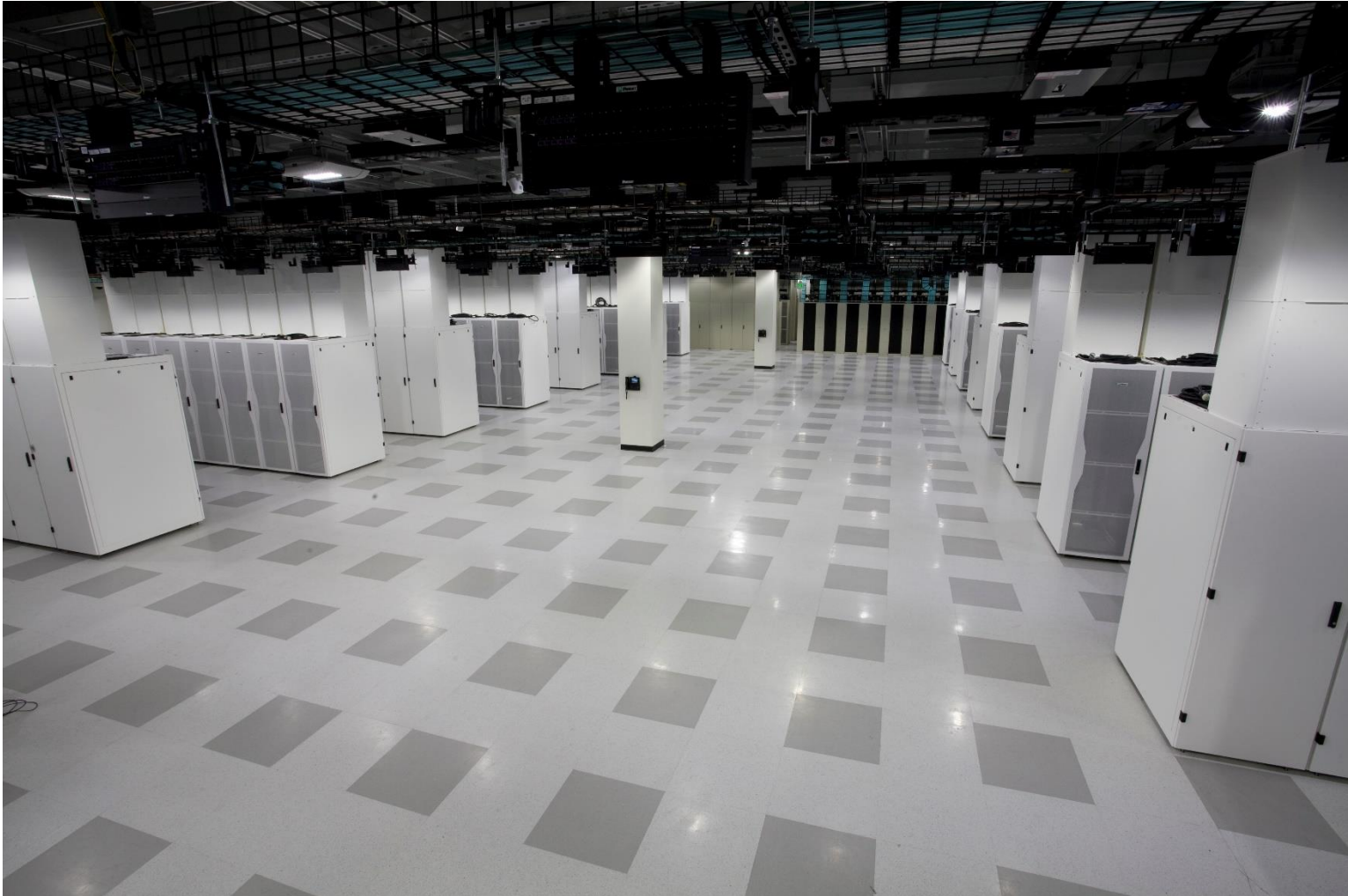
Cisco's Data Center in Texas
