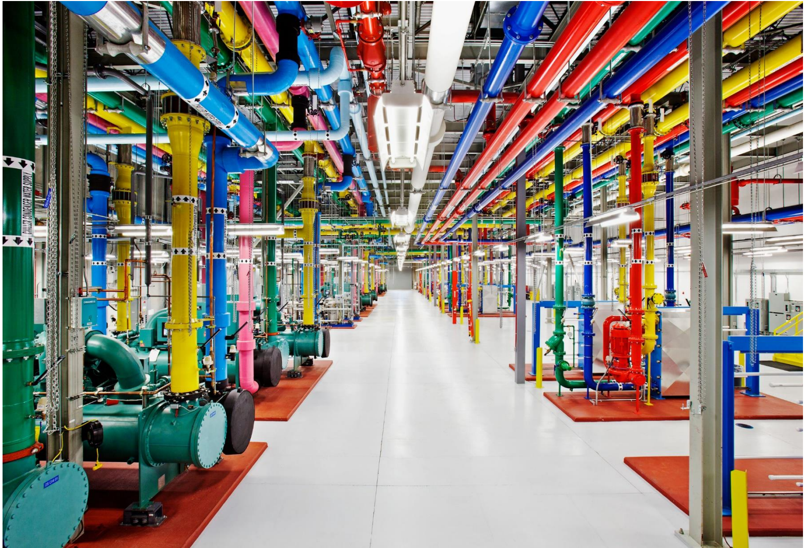
2017-01-17 Google's Data Center in Georgia
