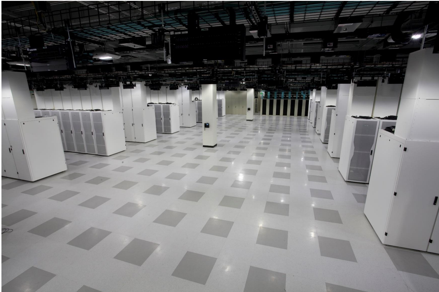
2017-01-17 Cisco's Data Center in Texas
