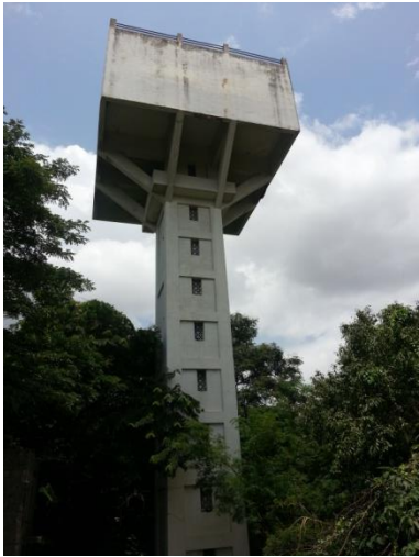
TPH (near Mechanical)
